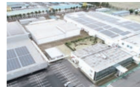
Solar power system at Tsukuba Plant
